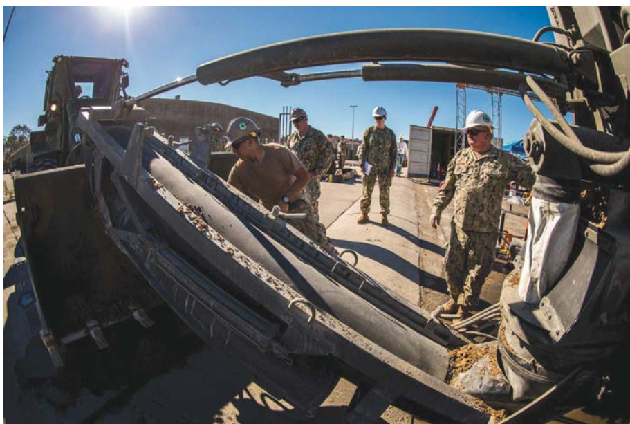
Marines, Sailors, and Soldiers work together to make concrete. (Photo by LCpl Betzabeth Galvan.)
