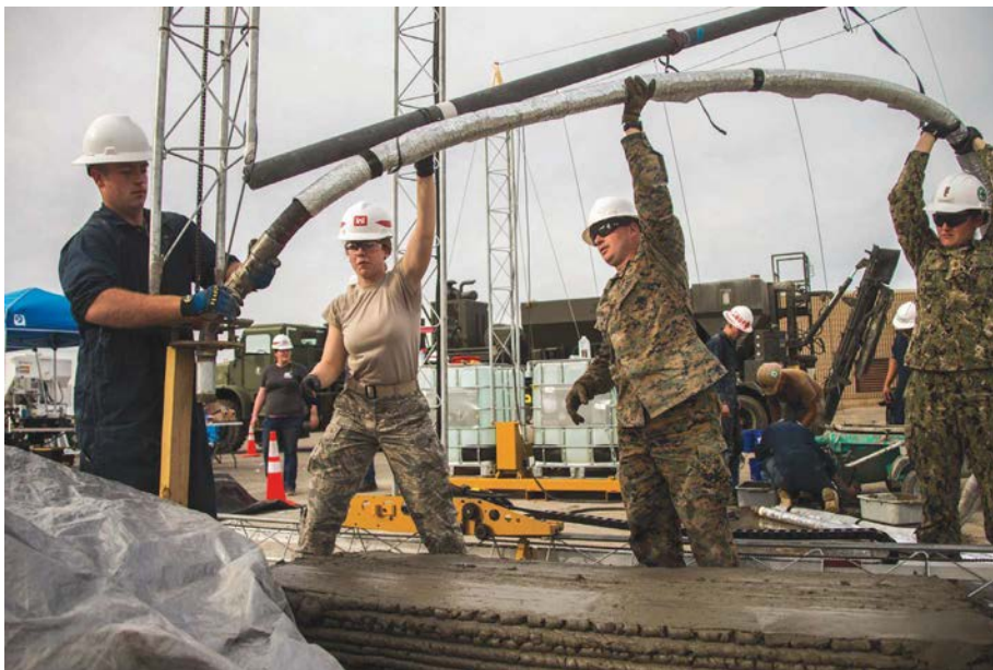
7th Engineer Support Battalion Marines and Naval Mobile Construction Battalion 5 used the automated construction of an expeditionary structure printer to conduct 3D printing. (Photo by LCpl Betzabeth Galvan.)
